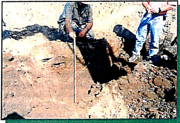
Figure 3-7: Using a backhoe, small trenches are dug perpendicular to the centerline of the historic ditch/canal. Samples are collected from the side walls and floor of the trench at 2-foot intervals (or on a 2-foot grid) or where the characteristics or strata of the soil change.
