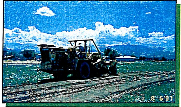
Figure 4-10 : A Cat SS-250 is utilized to deep till to an 18-inch depth.
