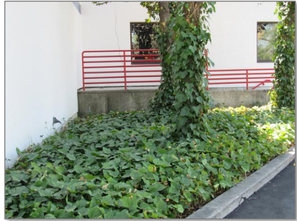
Figure 7: Downspout disconnected from parking lot
