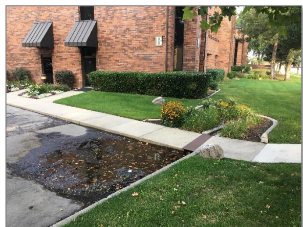
Figure 11: Standing water after a rain event at a bioretention BMP.
