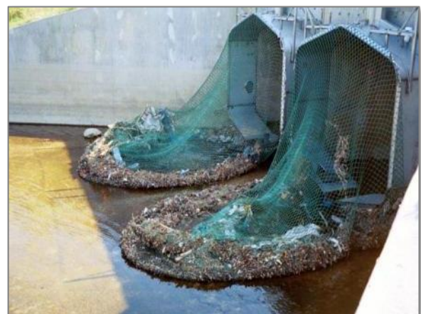
Figure 5: End-of-pipe trash netting
